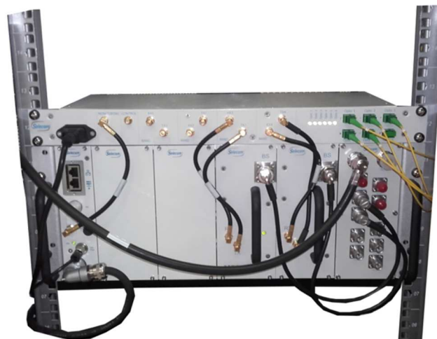
RF reception: Repeater rack and passive /optical rack
